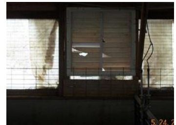
Fans need repair?
